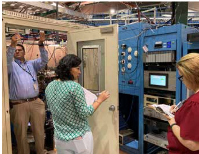
Amin M. Hamideh, Ji Young Wiley, and Melissa H. Esnault carry out an inspection on radiation interlock systems at the J. Bennet Johnston, Sr., Center for Advanced Microstructures & Devices (CAMD).
